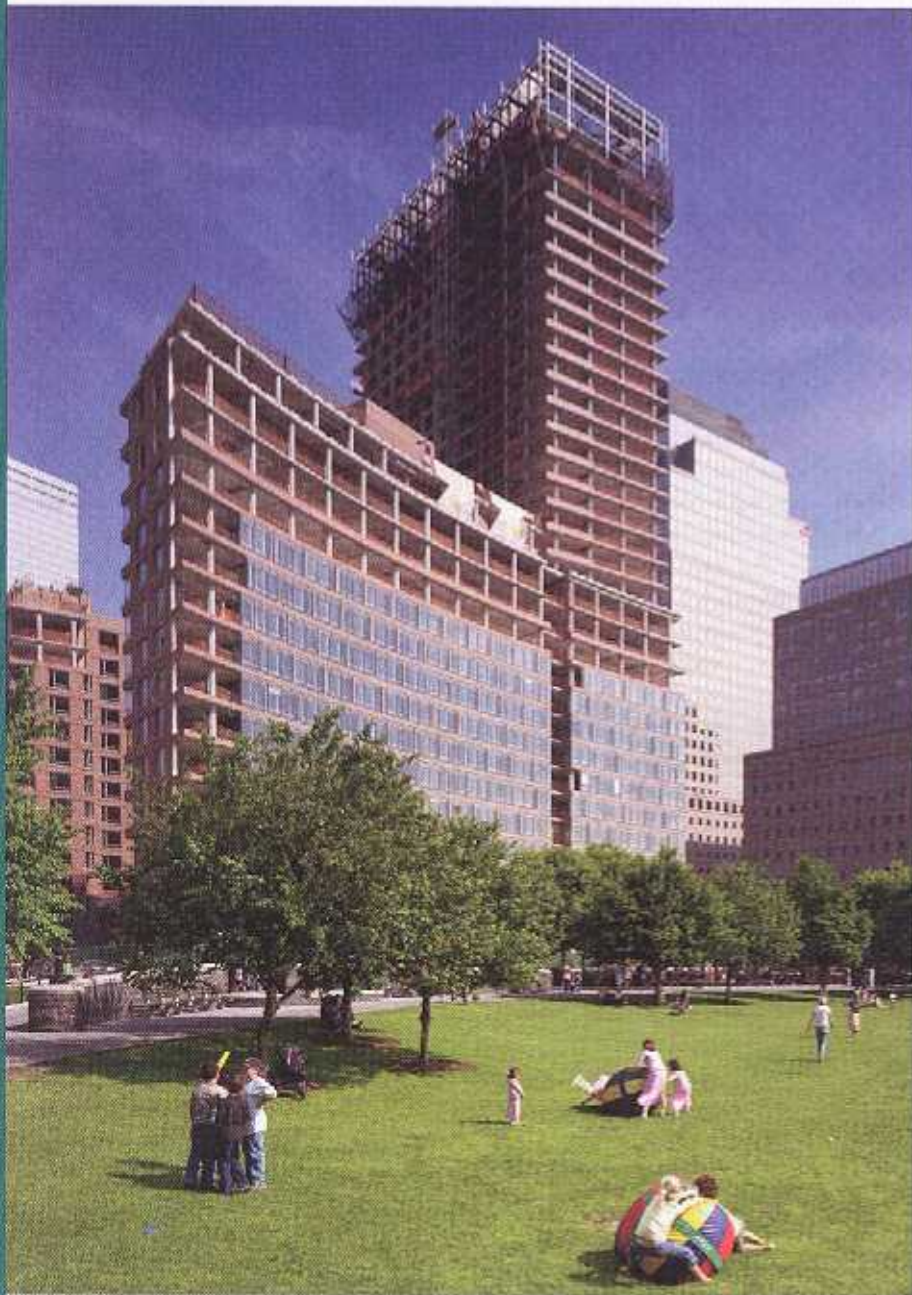
The Sheldrake Organization is aiming for LEED Platinum certification on Riverhouse at 1 Rockefeller Park in Battery Park City. However, the luxury condominium was also designed to appeal to tenants for whom eco-friendliness is a secondary consideration.
